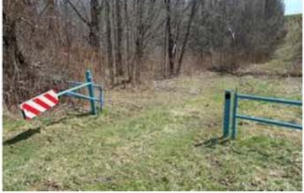
A gate meant to keep vehicles off a National Fuel pipeline right of way off Henderson Road in Millcreek Township was broken this spring. ATVs and other vehicles regularly travel the right of way, property owners said. CONTRIBUTED//ERIE TIMES-NEWS
